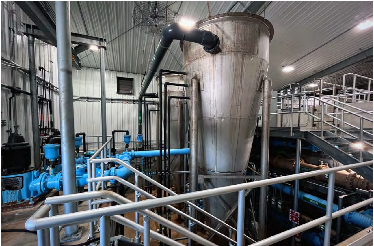
Water filtration at the Water Treatment Plant.
